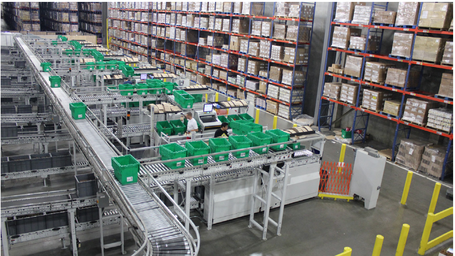
The good-to-person workstations are arranged in one zone adjacent to the Multishuttle sub-system.
