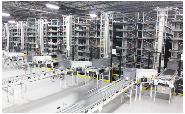
The Multishuttle sub-system serves as an inventory staging system and "pick engine."
